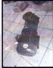
Bomba recalque M2
